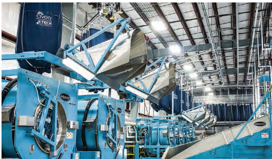
We are leveraging our existing infrastructure, such as our commercial laundry facility in the oil sands region, to drive incremental third-party revenue opportunities.
